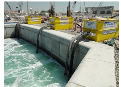
Settling tanks discharging into the sea.
