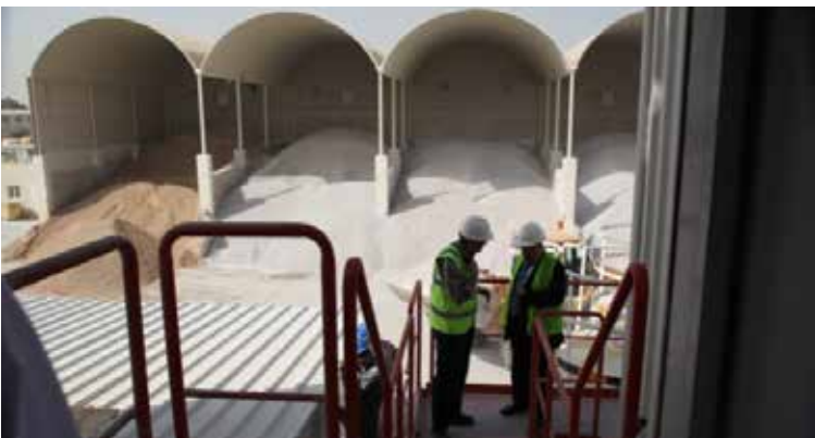
Covering raw material storage areas can reduce the generation of wind-blown dust.
